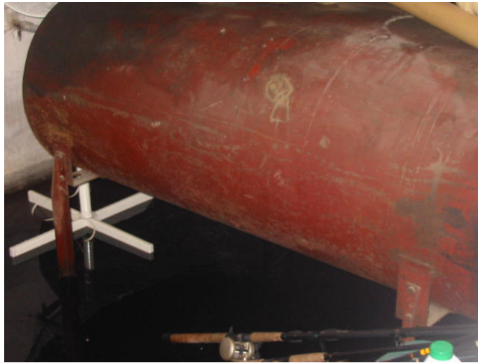
Figure 1. Release of heating oil from the tank
