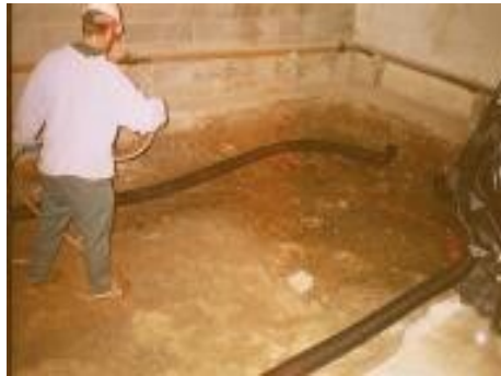
Figure 2. First application of biodispersion product after wetting the soil with municipal water. Black air vent tubes are seen in the background.
